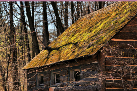
Roof covered in moss
